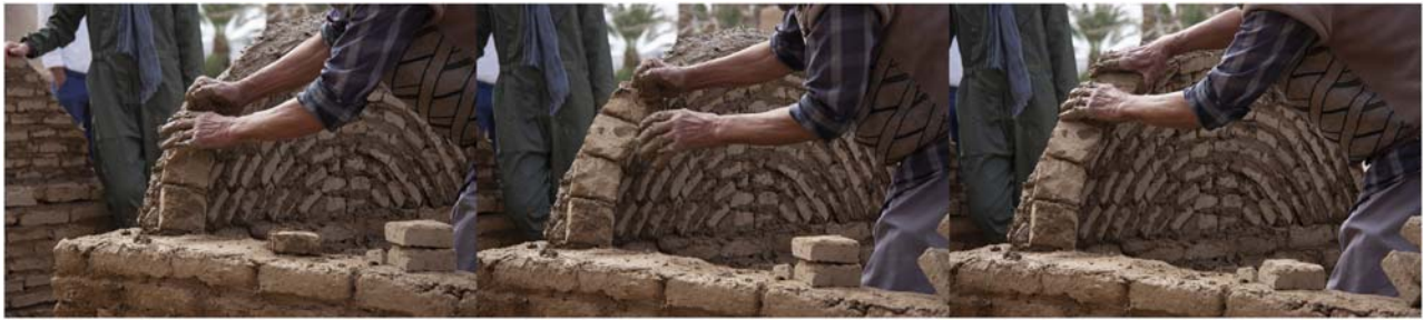
Figure 11. Ostad Ali during the construction of a 1:2 model of a sitting vault in a workshop in 2018.
