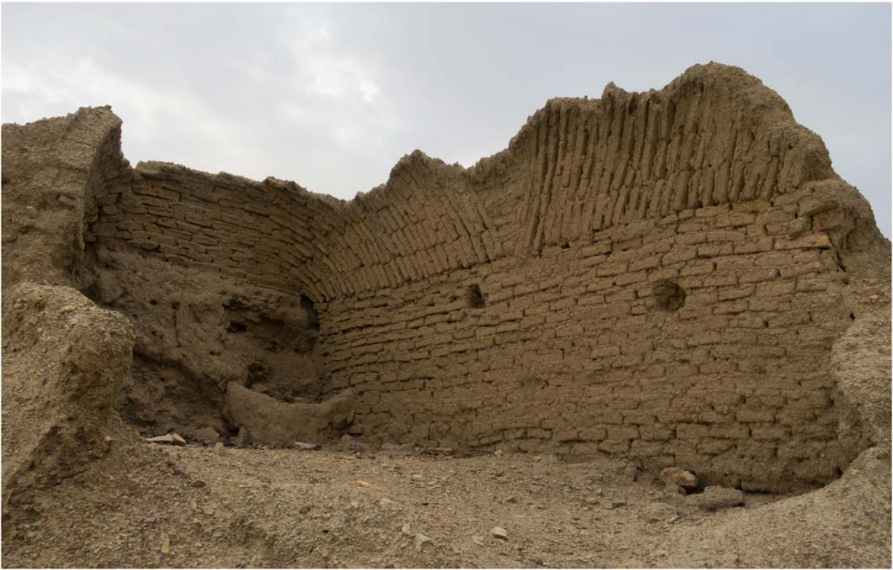
Figure 9. A sitting vault with different pitched-brick dispositions; Chiruk, a village near to Esfahak.
