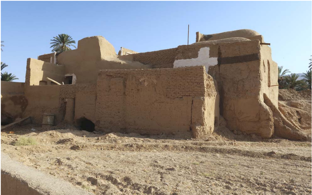
Figure 17. Abandoned house (same as the previous photograph) in the process of being restored, September 2019.
