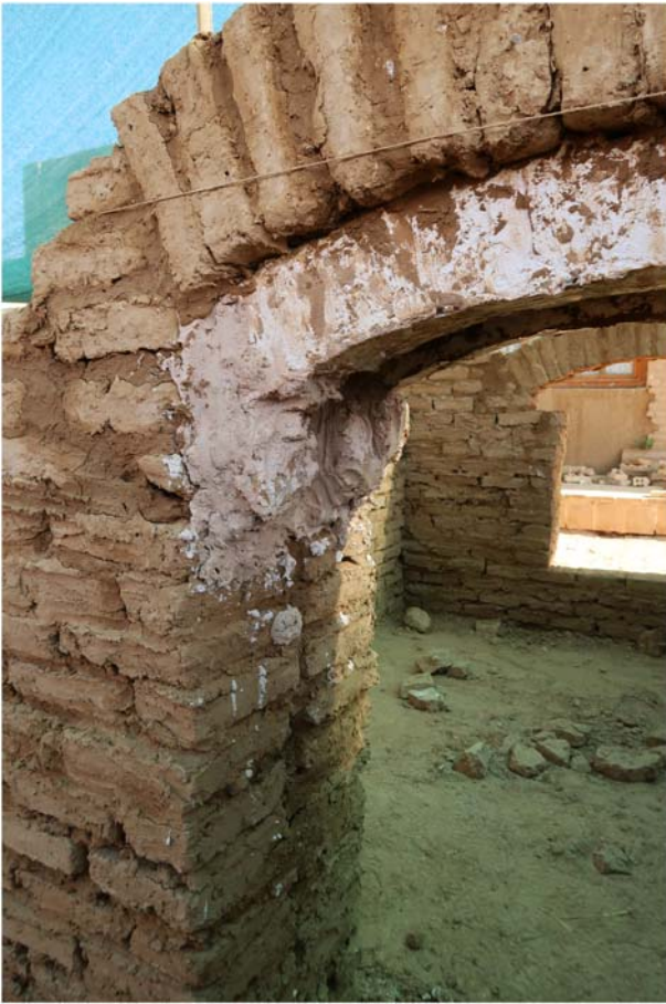
Figure 15. The use of a gypsum centring for the construction of a rumi arch on a door.
